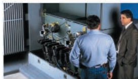
COOPER Power Systems
